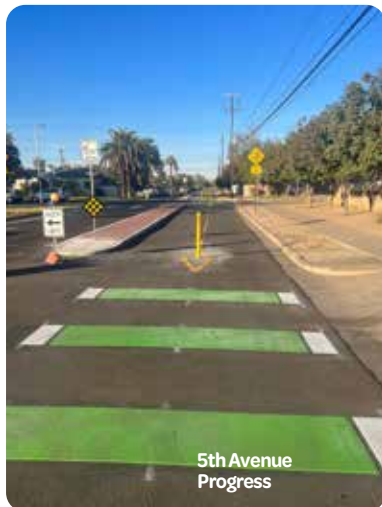
Willo resident Carl Schurtz (Encanto) joins the construction effort, if only in spirit!
